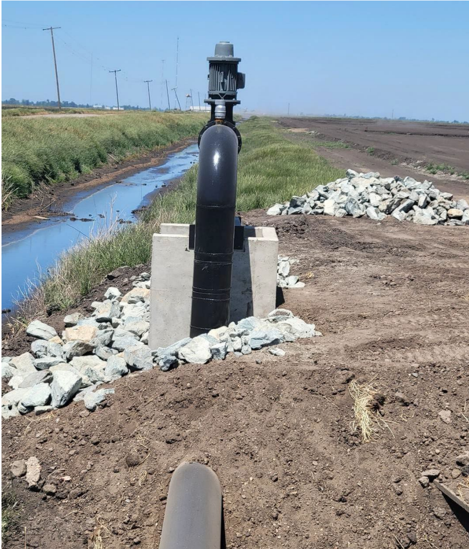
Figure 9.2. Completed Water Quality Improvement Project at Staten Island (Site 1), Water Recirculation Pump.
