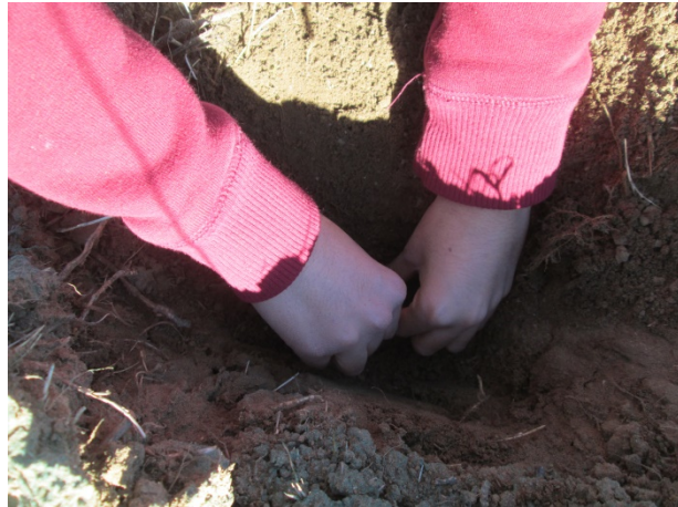
Figure 2. Student installing drip irrigation lines at the Ulatis Creek habitat restoration site.
