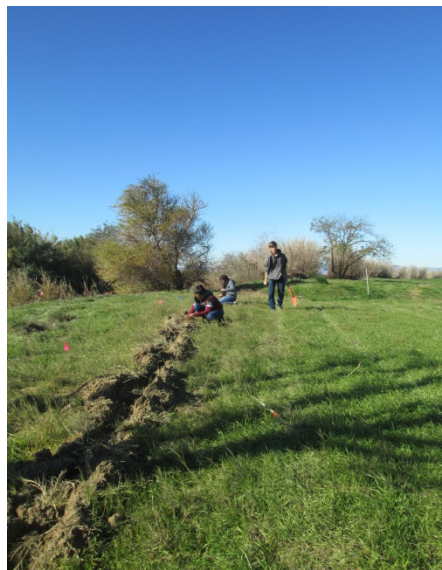
Figure 3. Ulatis Creek habitat restoration site showing SLEWS students installing drip irrigation lines.
